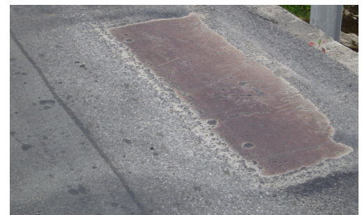
Steel Plate Bridging Failed FRP Deck Panels
